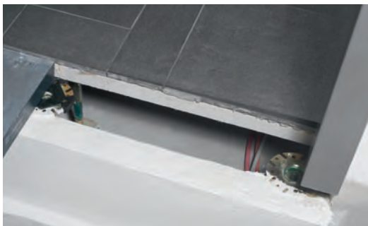
Composite access floor in shower unit covered with ceramic covering
